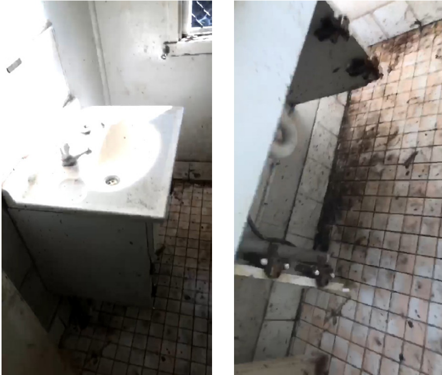
Figures 6 and 7: Bathroom on 4 June 2019 331
