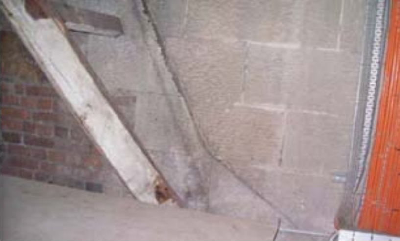
Figure 109: Portion of the attic wall showing the stone facing of the George Street wing with the mark of the flashing of the rear section of mansard roof which was demolished for the Alice Street wing
