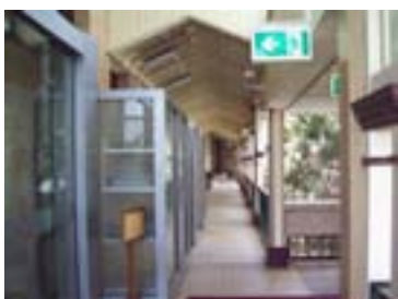
Figure 116: Glass doors added to a new entrance to the Alice Street wing (at left) leading from the Annexe. The modification of the verandah ceiling for ductwork is also visible.
