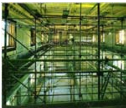
Figure 95: Restoration of the Legislative Chambers required scaffolding to be erected from floor to ceiling
