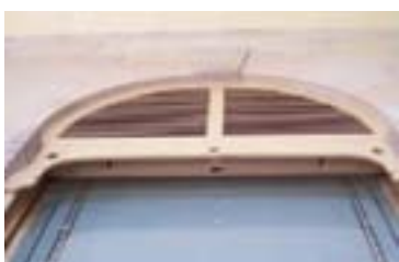
Figure 115: Marks of pulleys survive in the head of this blind in the George Street arcades. The parting beads in the jambs can also be seen. The valance is probably a later addition.
