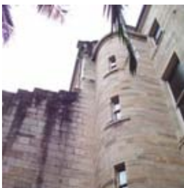
Figure 106: The circular reporters' stairs to the Legislative Council Chamber and the abutment wall to the rear verandah. The abutment would have formed the back wall of the south eastern wing.
