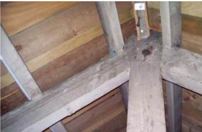
Figure 110: Ridge in the George Street wing. The gaps between the original boarding (the darker timber), which have now been filled, may relate to the laying of the original zinc roofing.
