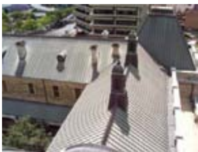
Figure 104: View towards the north tower. The new copper roof is sympathetic in scale to the original roof and cresting has been repaired. The 1895 fleches over the Assembly Chamber survive reclad.
