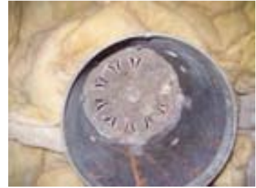
Figure 133: Possibly the remains of a 'sunlight' fixing in the roof space above the Council Chamber photographed from above
