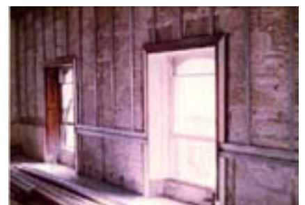
Figure 94: The old staff dining room, now the Billiard Room, where solid plaster was replaced with sheeting on steel battens to allow the introduction of services
