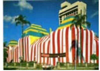
Figure 89: Parliament House being fumigated in 1980 to rid the building of the West Indian termite. About 16 km of reinforced plastic sheeting was used to stop poisonous gas escaping in the process.
