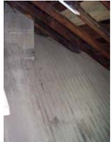
Figure 111: Early roofing survives in the attic at the back of the George Street wing where the Alice Street wing was added. It is not known why this is a different profile to the original samples.
