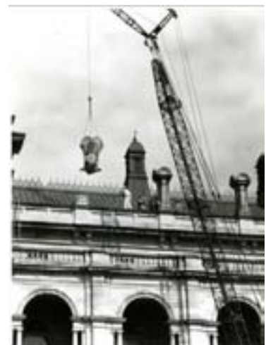
Figure 80: Removing pinnacles from the parapet above the Legislative Assembly Chamber, 1966. Some pinnacles can now be seen along the western edge of the Speaker's Green.
