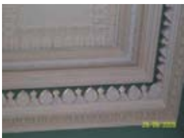
Figure 146: Cornice in the President's Office is more severe than the one in the Speaker's room
