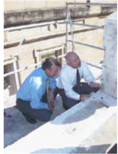
Figure 97: John McDonough, former Parliament House Property Services Manager, and Michael Hickey, Director of Corporate and House Services, inspecting the stonework
