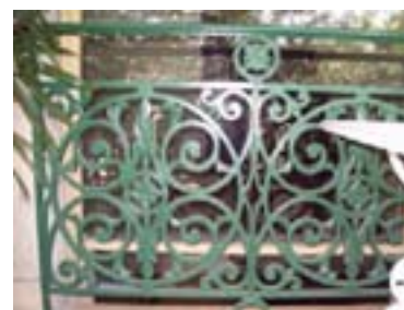
Figure 119: A section of original balustrade survives on the Alice Street verandah at first floor level, reused as a safety barrier for the window over the stairs
