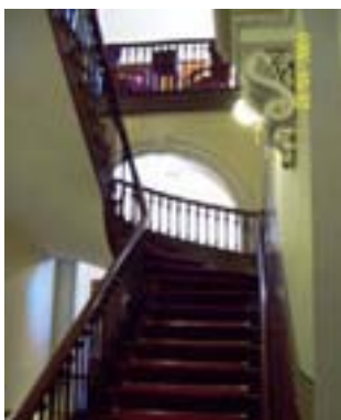
Figure 174: Staff stairs in the north tower, the balustrade against the archway is cast aluminium whilst the remainder is the original cast iron
