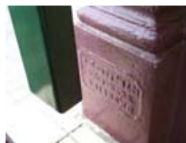
Figure 120: Manufacturer's mark 'J.W. Sutton & Co. Engineers Brisbane' on the bases of verandah posts at second floor level on the Alice Street wing
