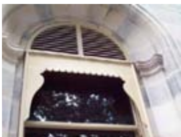
Figure 114: Remains of louvred shutters and the valance for a canvas blind on a window in the east tower. The valance appears to have been retrofitted and has a lead flashing at the top.
