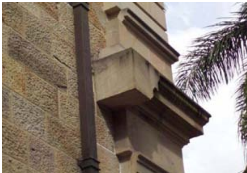
Figure 107: String course on the east tower prepared for adding the south eastern wing, which never eventuated
