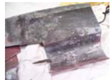
Figure 24: Sample of roofing viewed from below, showing the interlocking system of nails and slots. The nails were soldered to the underside of the zinc.
