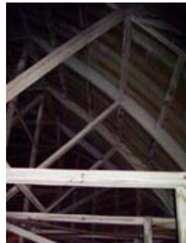
Figure 113: Curved pine rafters form the shape of the mansard roof over the main entrance. This was repaired in the 1980s renovations.
