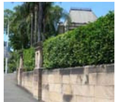
Figure 201: New walling at the western corner of the site looking north east
