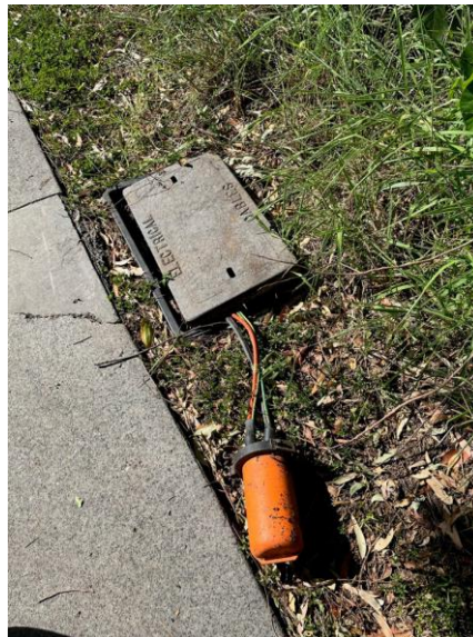
Exposed wires left next to public footpath after copper theft. (Carseldine, Brisbane 2023)
