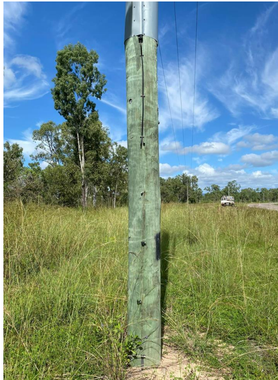
Power pole with stolen section of copper neutral earthing wire (Black River, Townsville)
