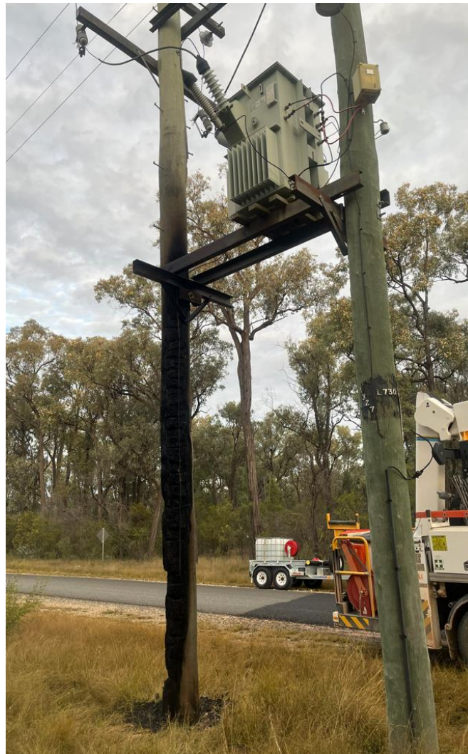
Fire-damaged pole caused by the stealing of the copper neutral earthing wire (Townsville)
