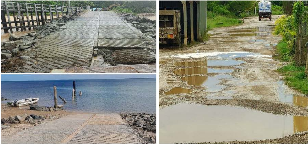
Figure 4: examples of the poor road and ramp infrastructure in Duaun Island and Saibai Island
