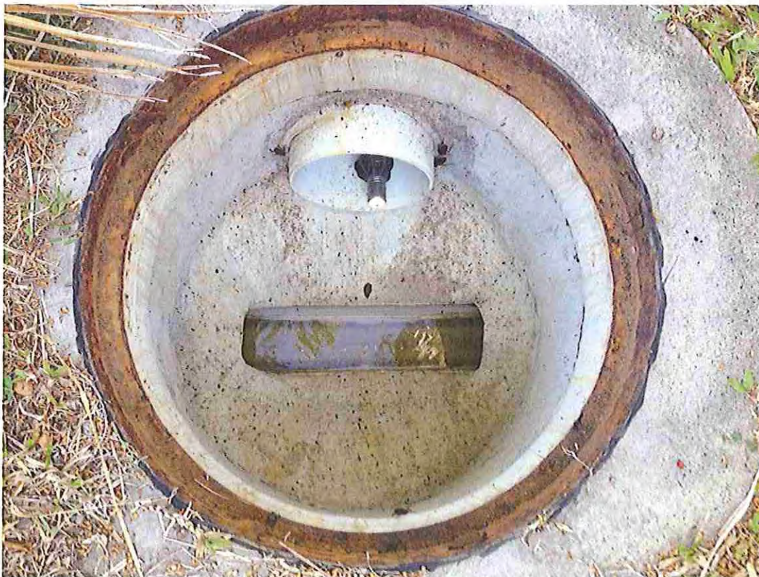
Inside sewer manhole, shows sewer opening and illegal pipe leading to stormwater drain (with drain camera inside)
