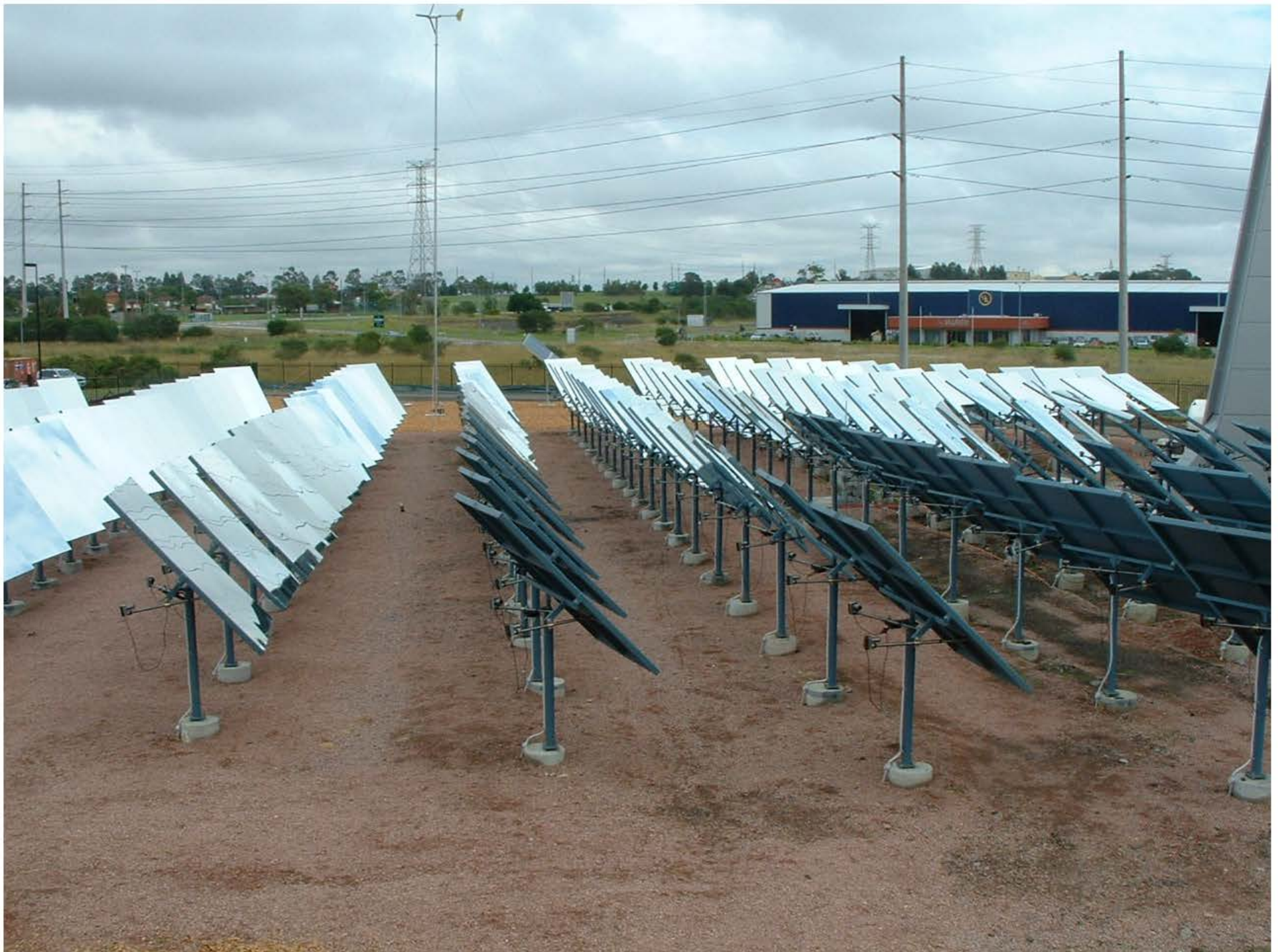
Similar heliostat array operating in Newcastle, NSW
