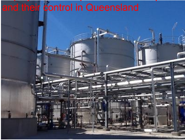
Figure 2: Beta Renewables Ethanol Plant in Crescentino, Italy
