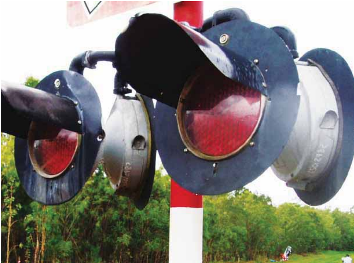
Figure 31: Close up of Rungoo LED light signals, individual LED's visible
