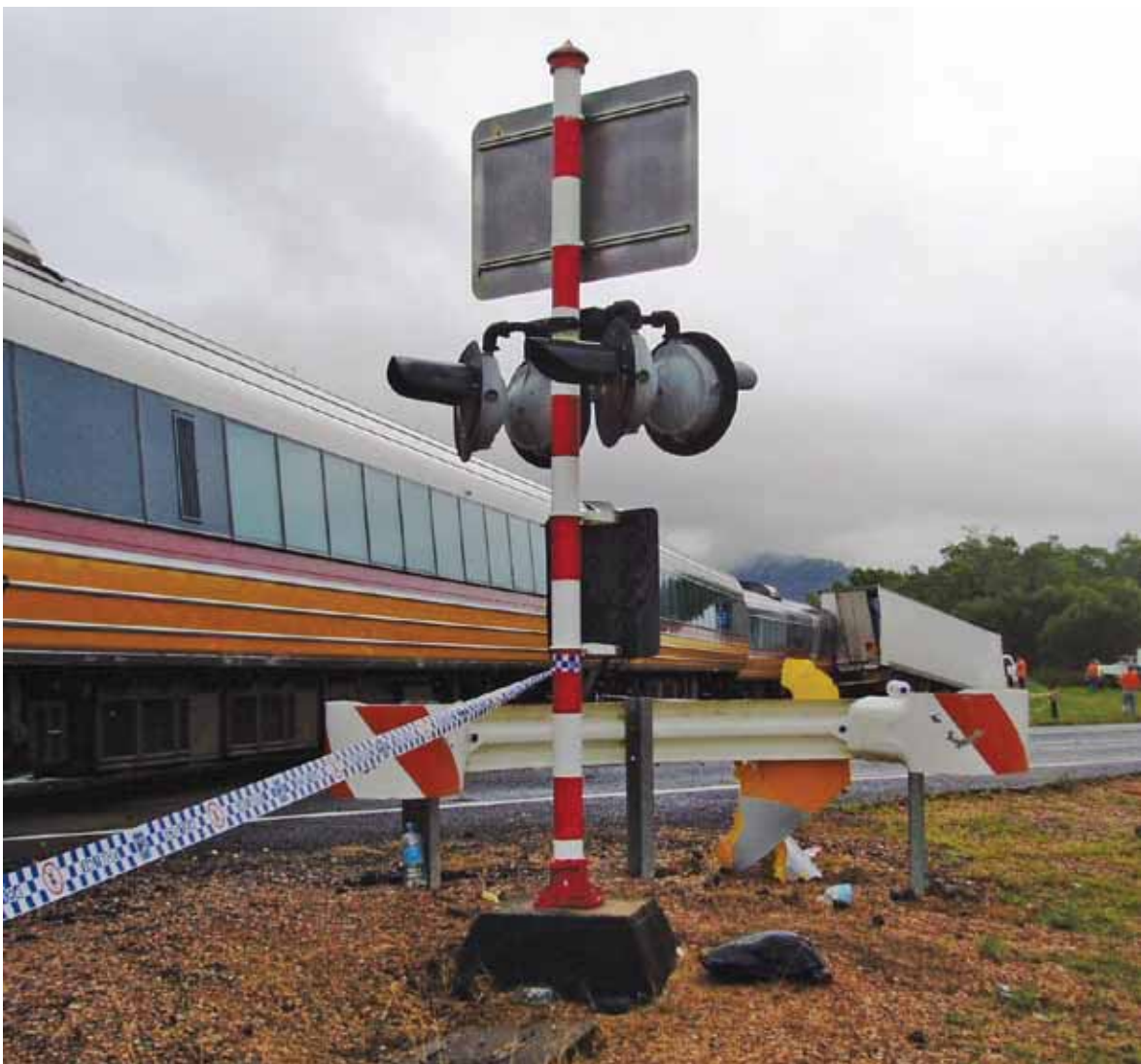
Figure 29: Rungoo level crossing signal assembly showing front (north) and back (south) warning lights
